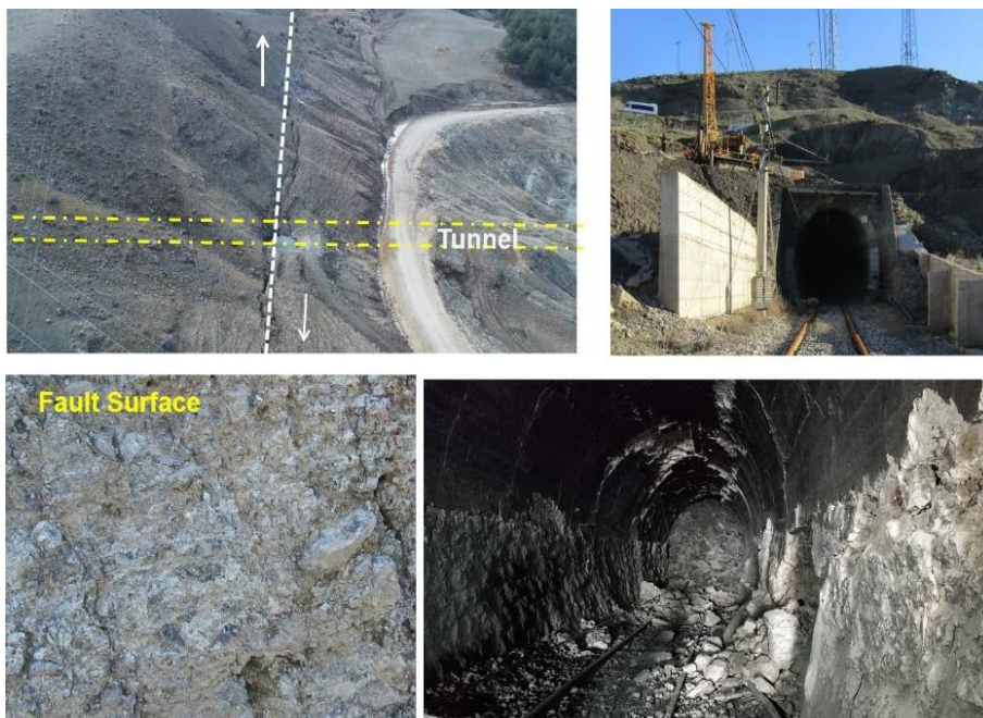
Figure 6. Damage to the Ozan railway tunnel by faulting
