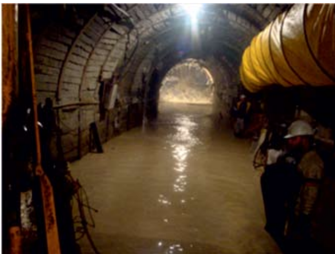
Fig. 9 : Flooded Tunnel with Seepage Water
