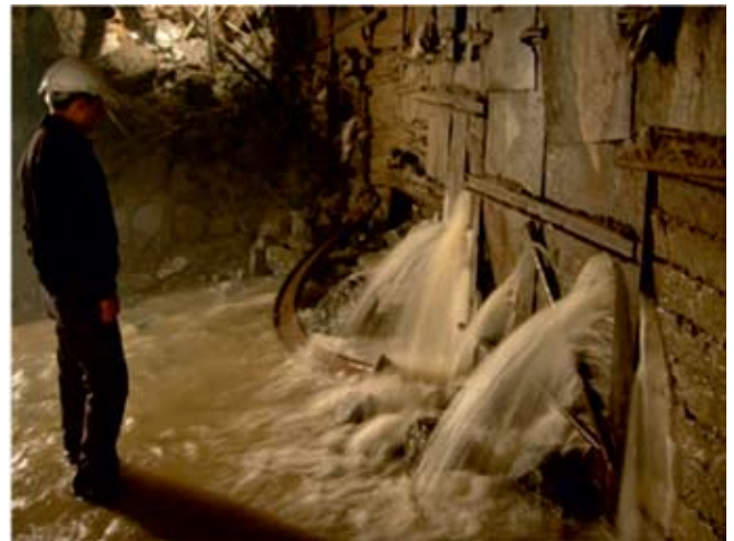
Fig. 11 : Heavy Seepage Water with Pressure
