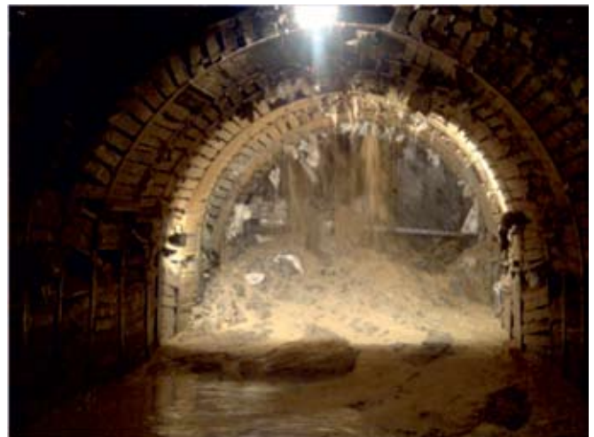
Fig. 1 : Heavy Inflow of Seepage Water
