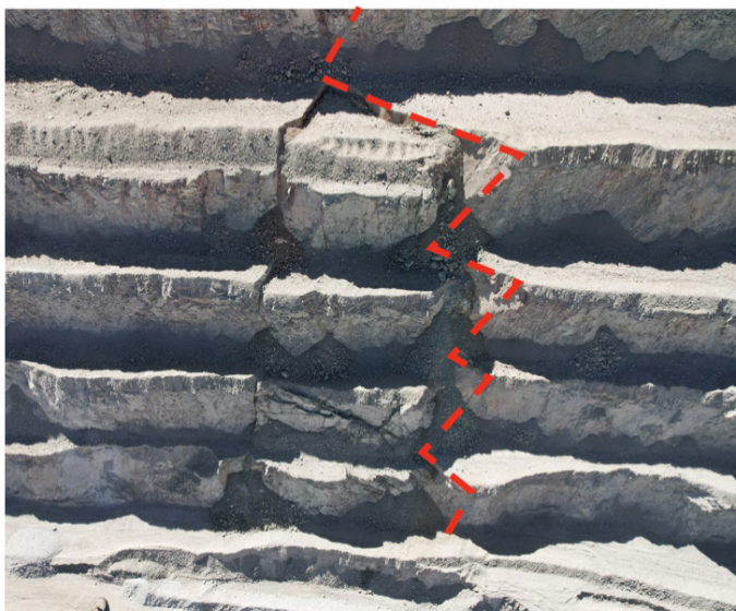
Fig 12. Example of a class of instability in open pit mines referred to as non-daylighting wedge. The instability occurs along the fault (indicated by the red dashed line).
