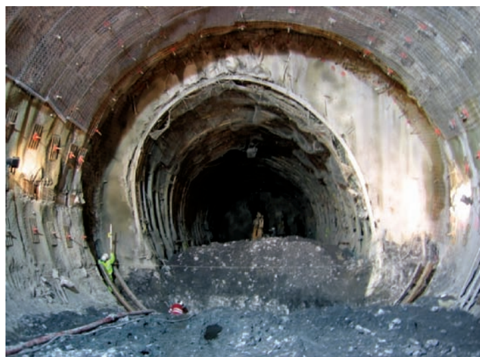
Figure 2. Very large convergence during the excavation of the Saint Martin la Porte adit for the project of the Lyon-Torino railway project
