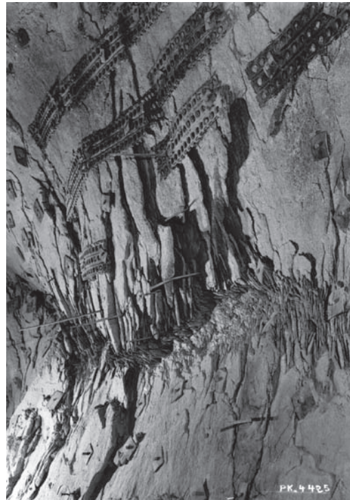
Figure 4. Heavy rockbursting in the Mont Blanc tunnel
