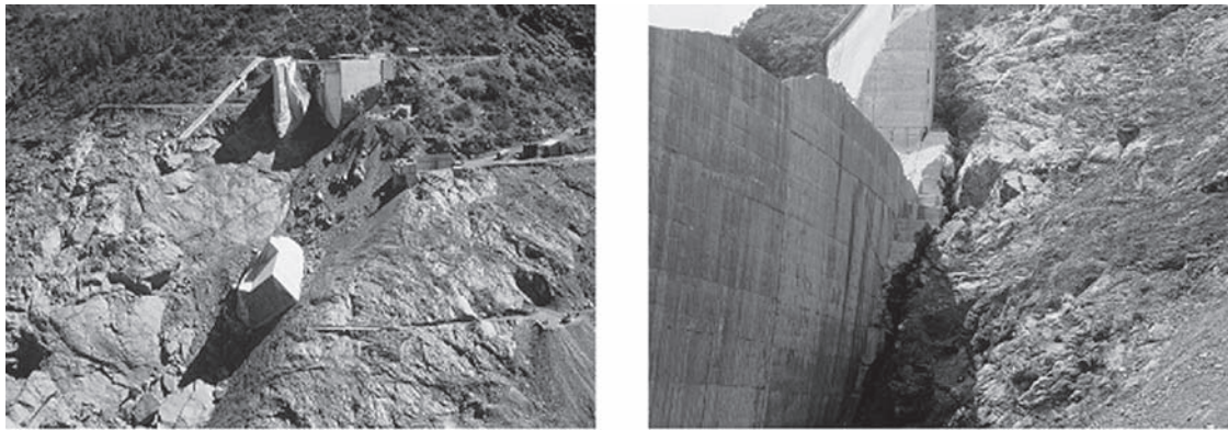
Figure 1. The Malpasset Dam Failure: left, the rock failure on the left bank abutment; right, the large fissure along the upstream abutment on the right bank
